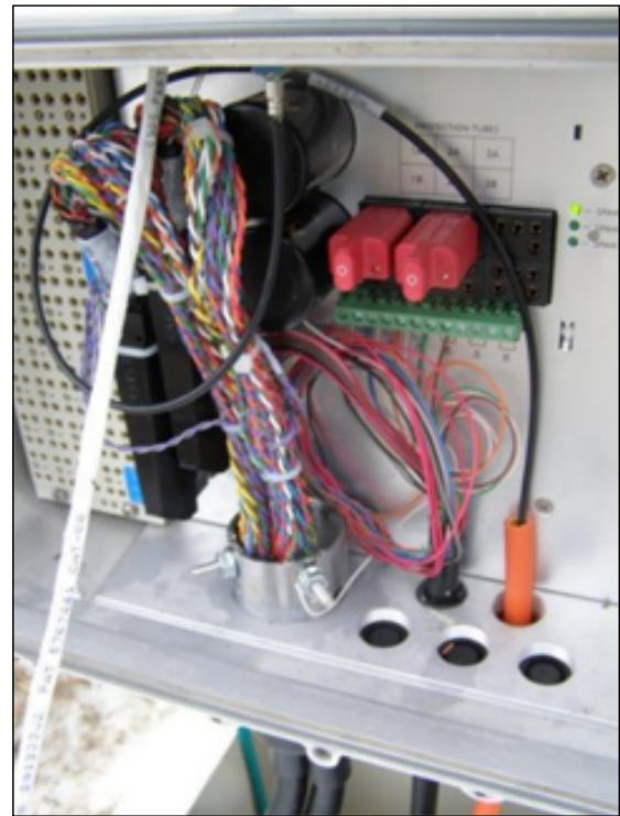
Figure 4 Typical DSLAM Terminal Strip
