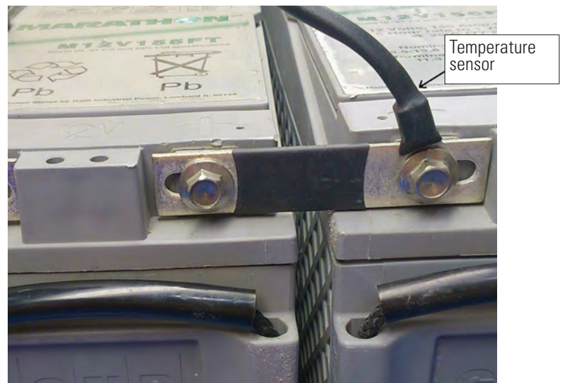
Figure 28: Battery temperature sensor, battery bay
