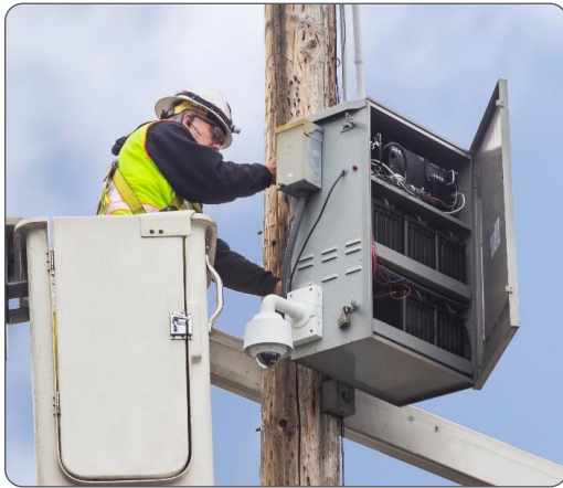
Figure 8 –Typical Broadband UPS
