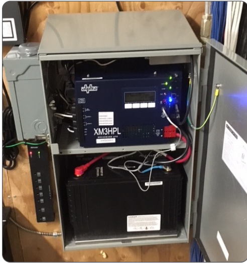
Figure 10 – Small Broadband UPS for Dedicated R-OLT Powering
